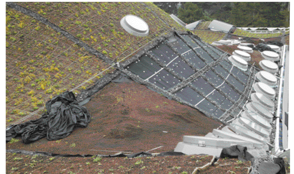
Peeled away view of the roof showing several layers of the roof system.
